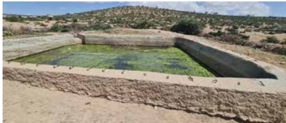
This previously derelict berkad in Qoolcadey, Somaliland was responsible for the death of five children. It was uncovered and the water was contaminated and deep enough for a young child to drown. Mercy-USA made major improvements to this berkad (feature photo above) that is now safely in use by the community.
